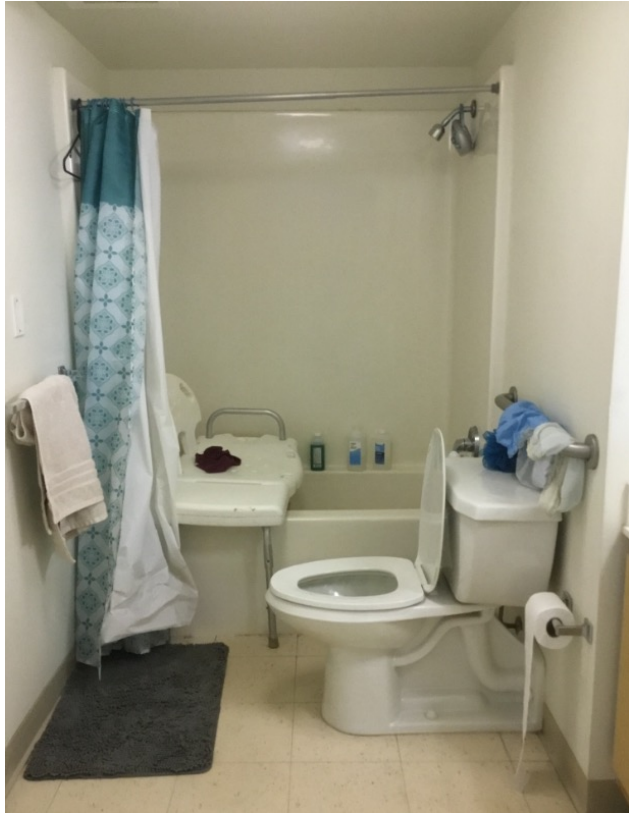
Pre-Compass: Toilet too low and no hand support. Using towel bar to transfer, but had pulled out of wall. Broken tub bench. Standard shower head made reaching all body parts difficult.
