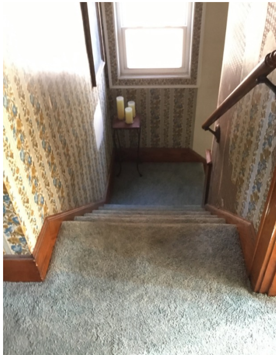
Pre-Compass: Unilateral railings. Current railing unstable, pulling out of wall when heavy pressure applied.
